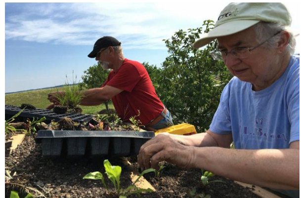
Board Member Peg Anzalone and member Willem Zijp working on the installation of the green roof at the education station
